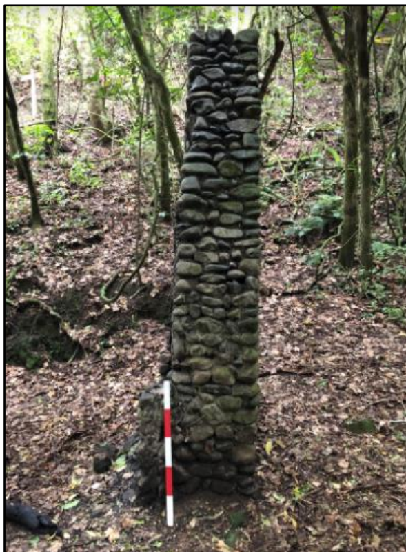
(Reference images of chimney situated in Jubilee Park taken by Nick Beynon 2020)
