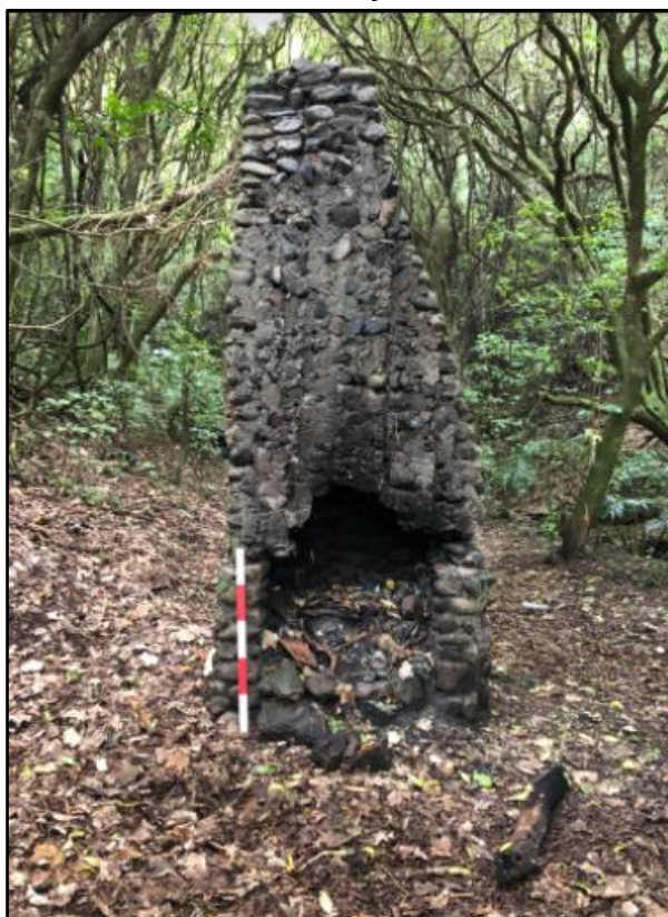
(Reference images of chimney situated in Jubilee Park taken by Nick Beynon 2020)
